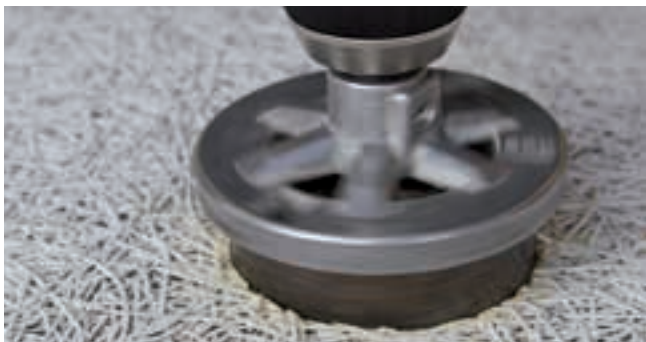
Drilling of a round aperture for a spotlight, with tile face side up.
