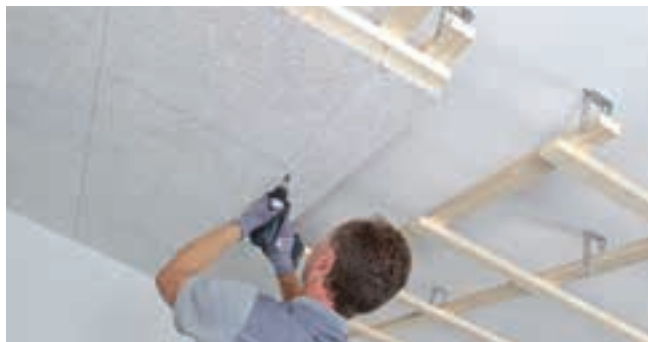
Exchanging the ceiling grid for the installation of modular lighting: Additional cross profiles and hangers required in the area of the exchange.
