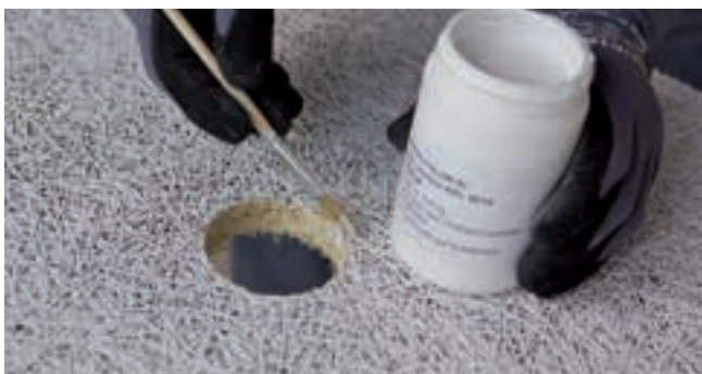
Cover cut edges with paint if these are not concealed by a cover.
